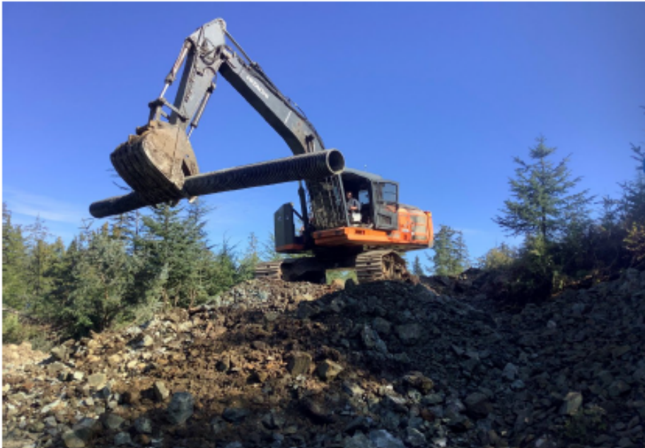
Culvert installation, Bay View timber sale on Prince of Wales island (Tom Chaney)
